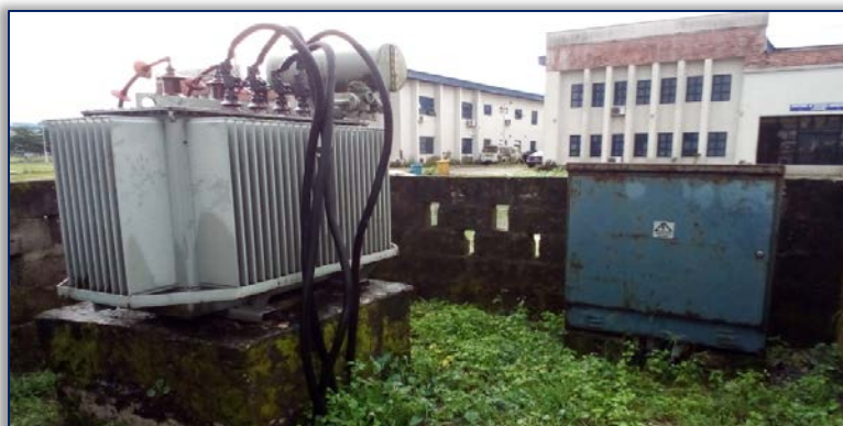
Figure 4. 500kVA, 11/415V Transformer situated at College of Technology
