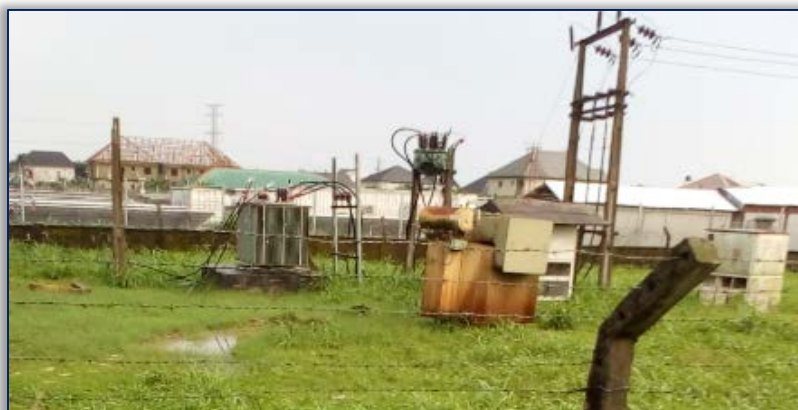
Figure 3. 2.5 MVA Transformer and its accessories
