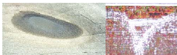
Figure 5. Void and pipe leakage detection
