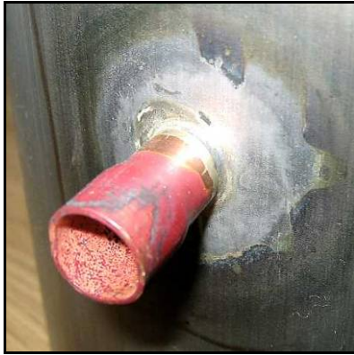
Fig. 2 Detail soldered joint copper mouthpiece of pressure vessel
