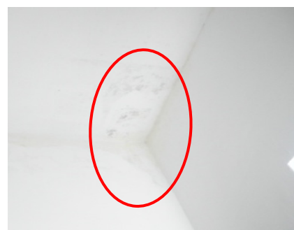
Figure 6: Water staining on ceilings
