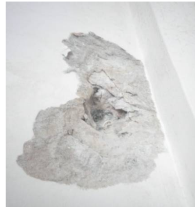
Figure 3: Plaster loose near to the store area at GTWHI building
