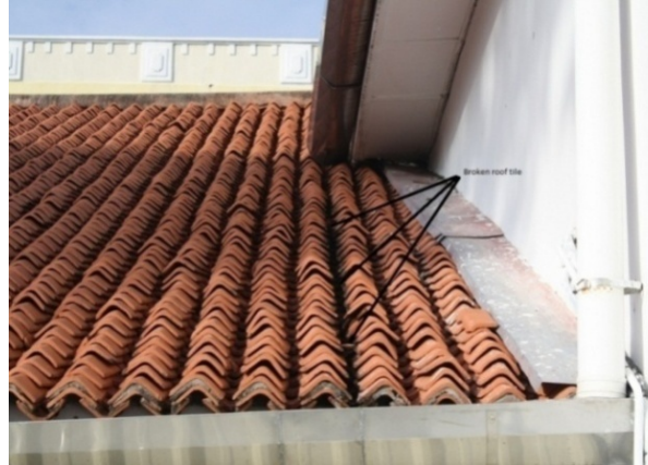
Figure 1: Slippery and broken roof at GTWHI building
