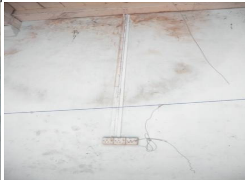
(ii) Water staining on wall
