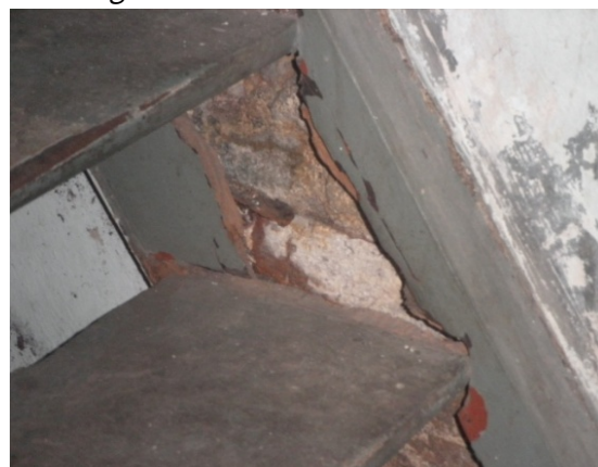
Figure 5: Timber decay appeared on the handrails of staircase
