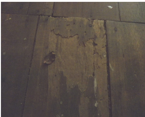
Figure 4: Termite attack can be seen on timber planks at the first floor
