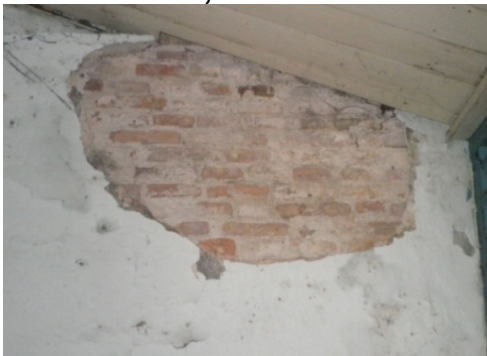
(i) Loose plasterwork of brickwork
