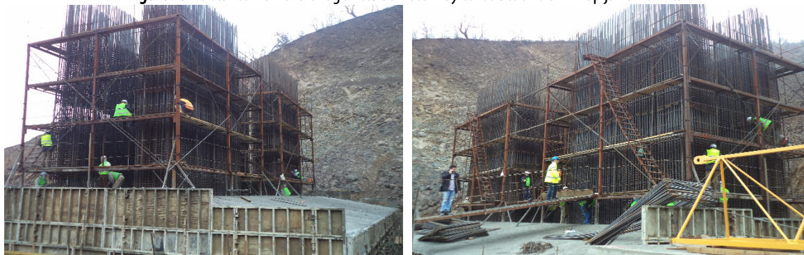
Figure 2. Scaffolds and ladders established on the bridge No.5 at Motorway construction Demir Kapija – Smokvica
