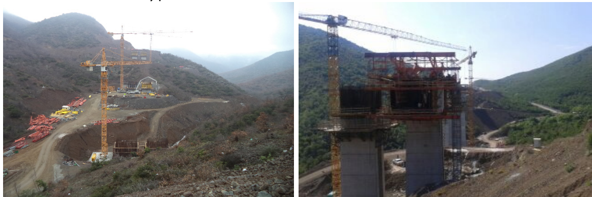
Figure 1. A distance view of a bridge No.5 at Motorway construction Demir Kapija - Smokvica
