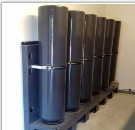
Figure 10. „Air bank” with two batteries of three bottles fixed to the wall [4].
