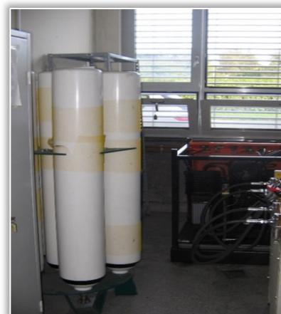
Figure 11. „Air bank” with two batteries and two bottles each, fixed to the floor [4].
