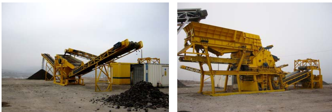
Figure 5. Instalation of slag treatment SPS Hunedoara
